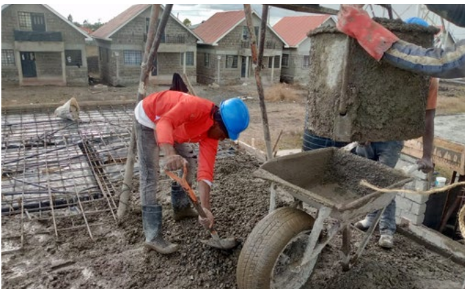
Above: Work on the slab for house 11 (above), opposite the first eight houses and facing the road to be built between them. The plot around the houses is for growing fruit, vegetables, herbs or keeping chickens
