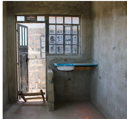
Above: Simple kitchen with a single cold water tap. Water is heated on a small LPG stove.
