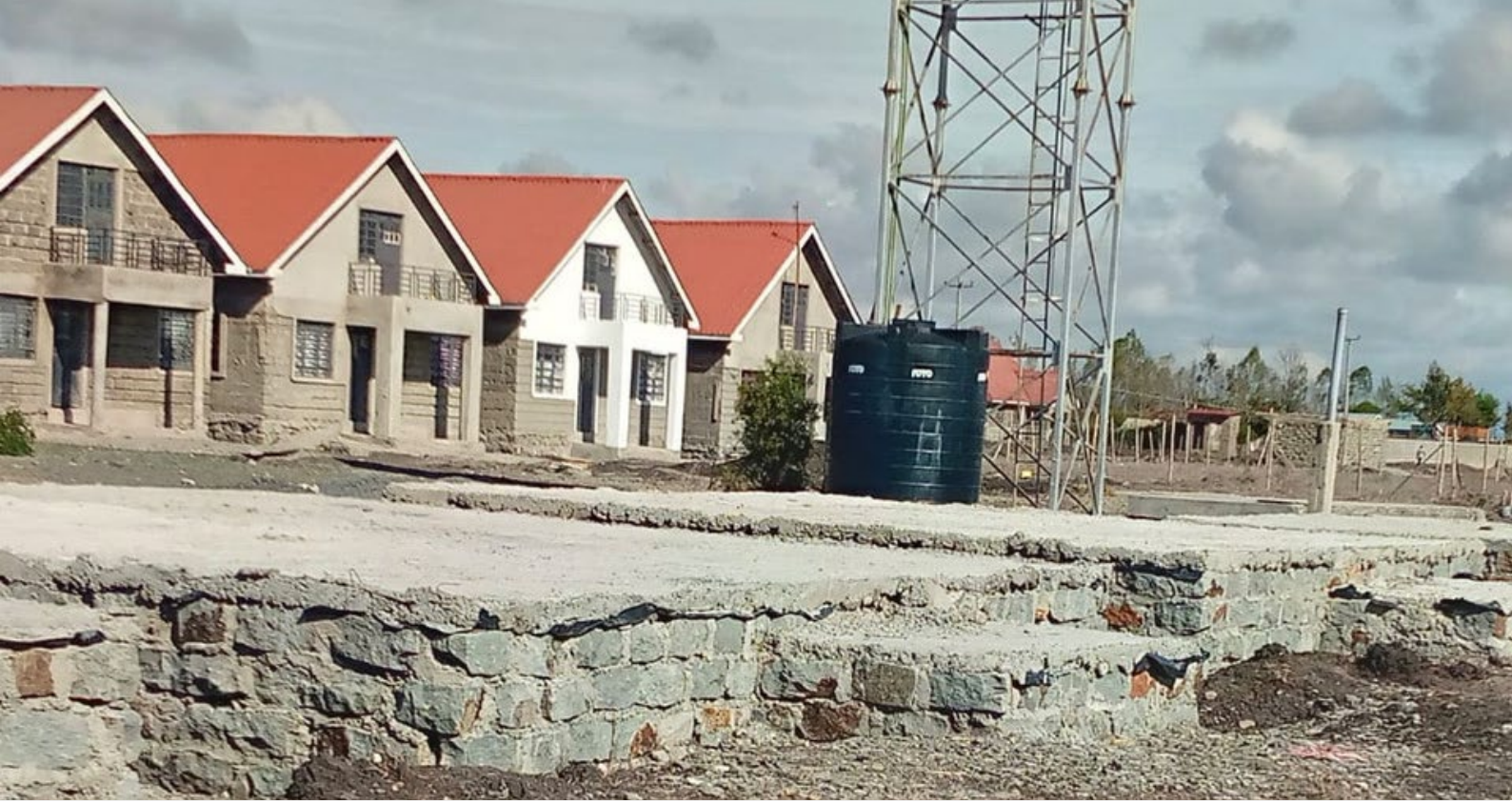
Above: view of the last four houses and the new foundations under construction - what a difference some paint makes.
